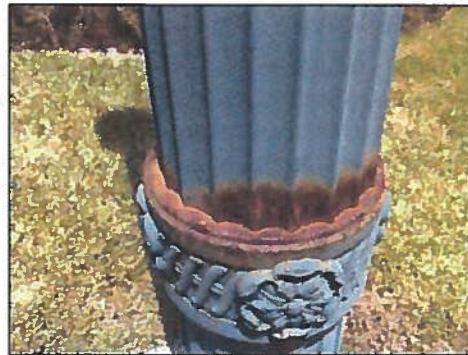
Lamp post-detail of corrosion, Image C.
