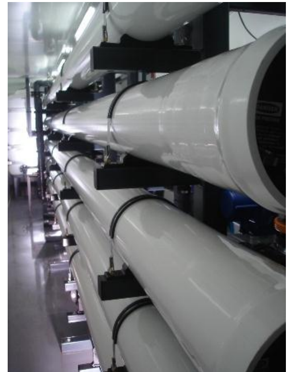
Reverse osmosis units, Noardburgum
