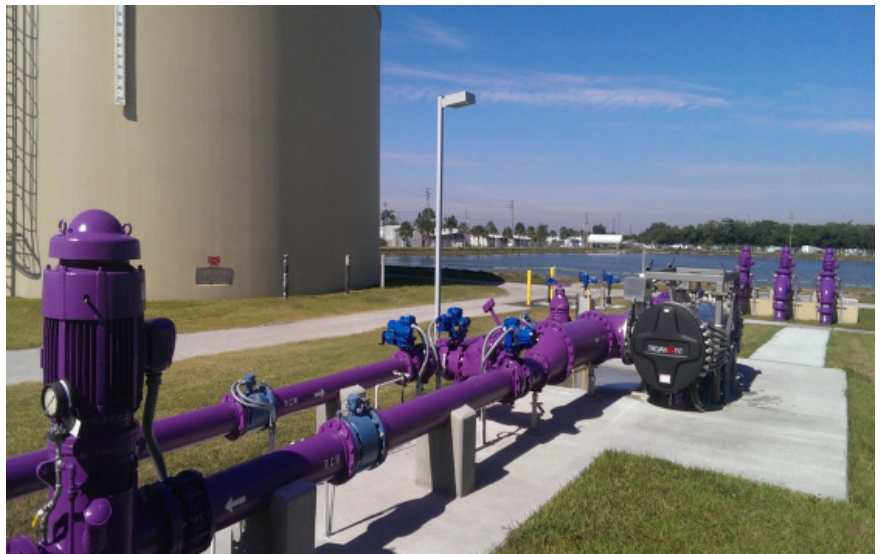
Inline UV System and Sodium Bisulfite Feed.
