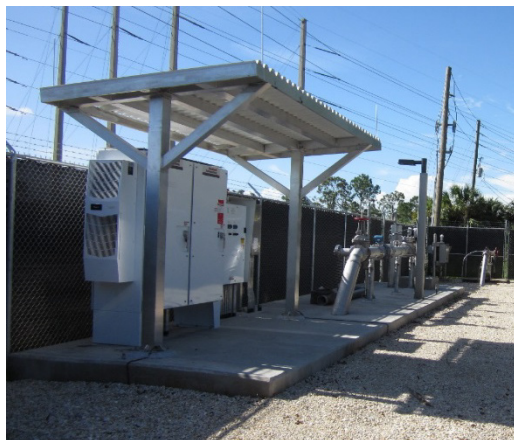
This project included engineering and hydrogeological design, including extensive geotechnical investigations for raw water line piping design and installation, as well as construction management for five new RO supply wells—similar to the City’s requirements for RO Well 8.
