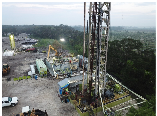
Construction of the Class V exploratory well was completed in January 2018 and an FDEP Class I Construction Permit Application is pending for the well to be converted to IW-1 for operational testing.
