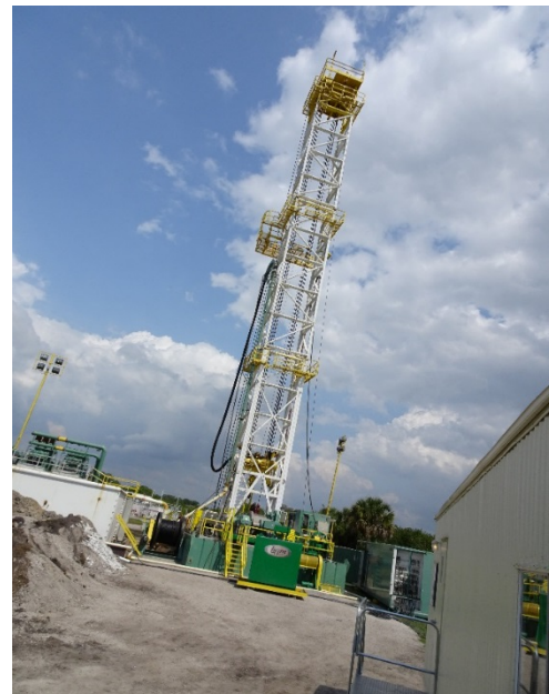
Jacobs helped secure an FDEP UIC Class V Test Well Permit, which involves recharging the UFA with reclaimed water containing less than 10,000 mg/L of total dissolved solids.
