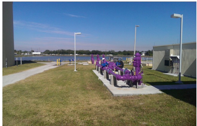
Completed Reclaimed Water ASR Wellhead facility with ultraviolet disinfection treatment and sodium bisulfite pretreatment.
