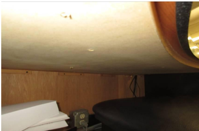
11 ) No evidence of suspect visible mold growth under the desks
