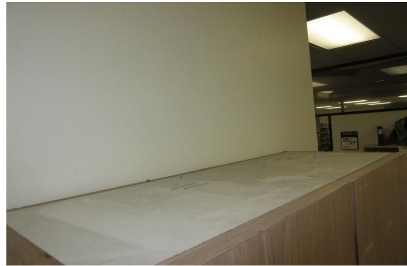
2) Upper cabinets revealed a significant layer of dust buildup.
