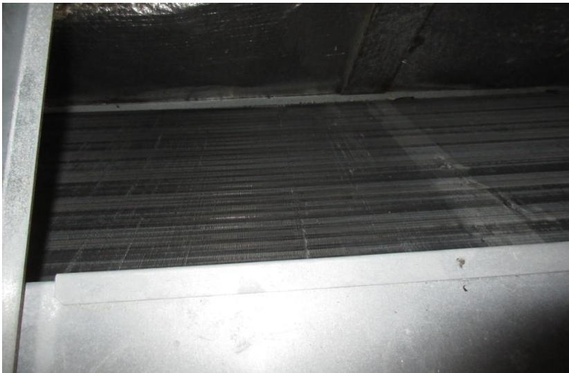
23) The upstream side of the coil appears to be in good sanitary condition.
