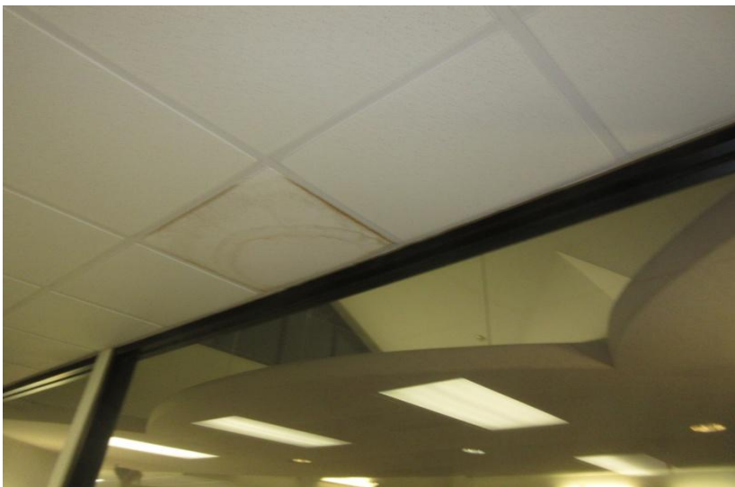
3) Ceiling tiles at the wall between the Workroom and Lobby revealed significant water stains.
