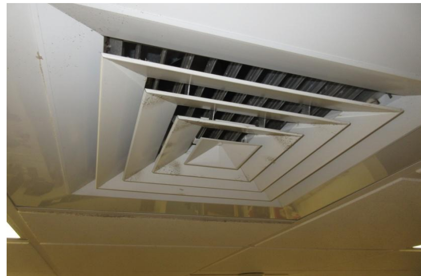
4) View supply grille reveals ghosting.
