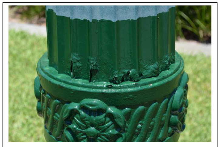
Detail of green paint covering corrosion
