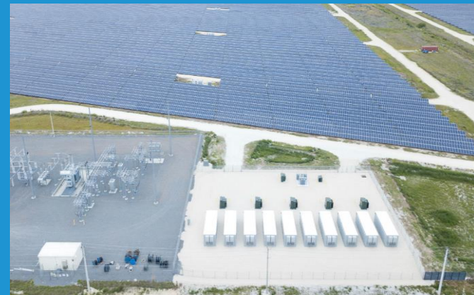
Battery Storage at Babcock Ranch Solar Energy Center
