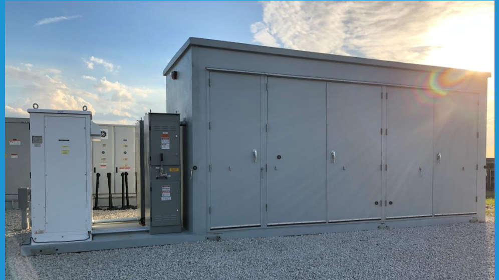
Battery Storage at Citrus Solar Energy Center
