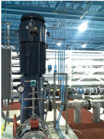
Figure 3 – Membrane Feed Pump
