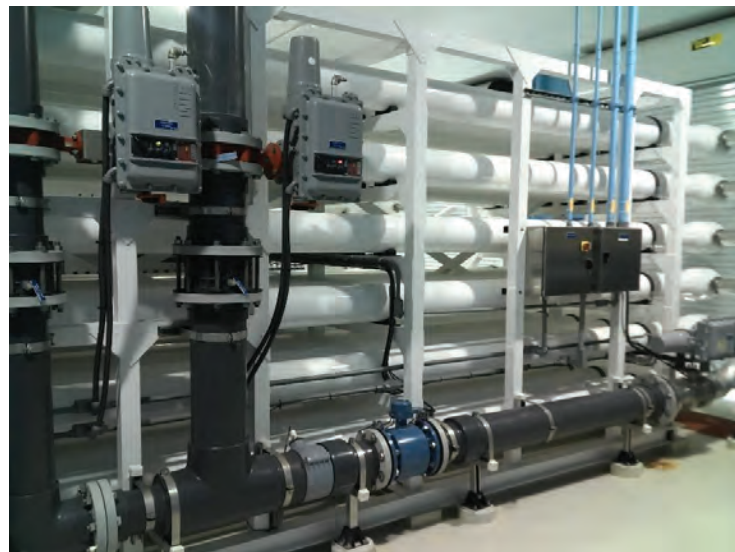
Figure 4 – RO Membrane Skid
