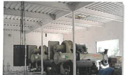
RCAD - Chiller Pumps
