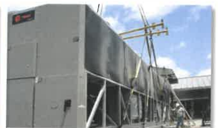
SBSC- Oak Park Chiller
