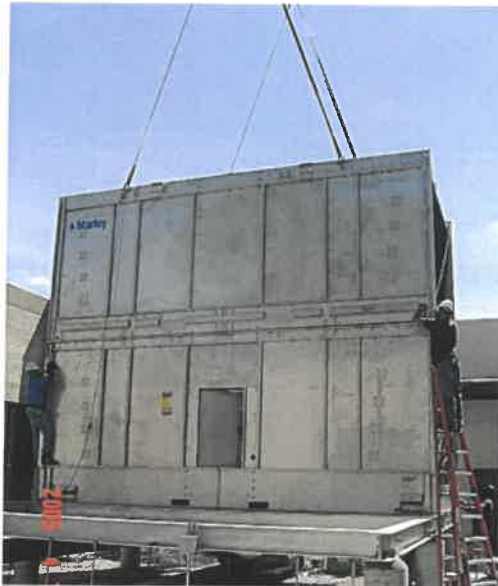
RCAD-Air Cooled Chiller Tower
