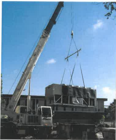
SBSC- Southside Elementary Chiller
