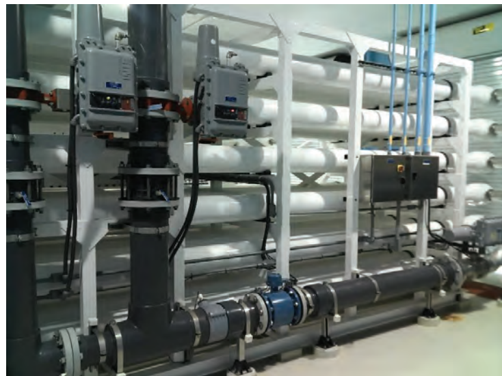
Figure 4 – RO Membrane Skid
