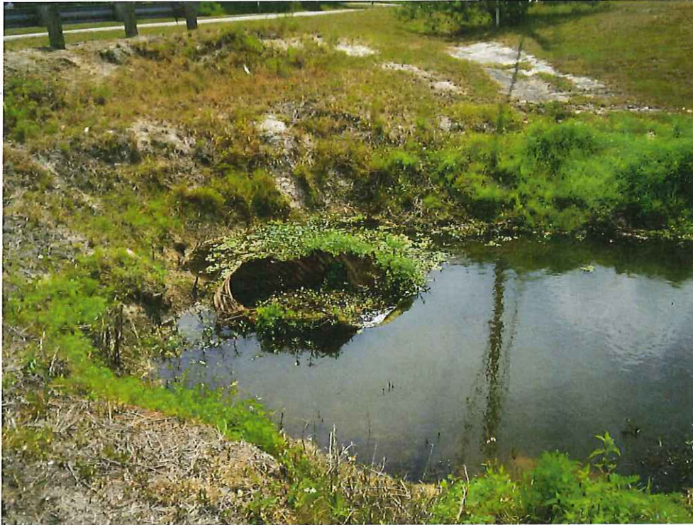
Old Drop Structure WCS 133 - 45 Degree Angle Corrugated Metal Pipe Drop Pipe Severely Corroded
