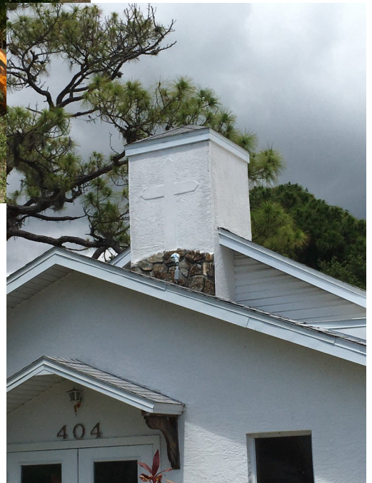
Detail of steeple where cross lites have been covered by addition.
